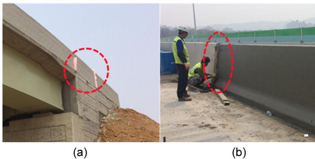
Fig. 1 Expansion joints installed in (a) bridge railing and (b) concrete median barrier
